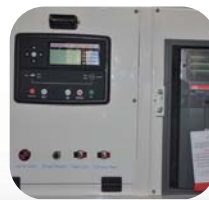
Control Panel & MCB
